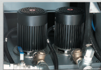
直立式泵浦 Vertical coolant pumps
